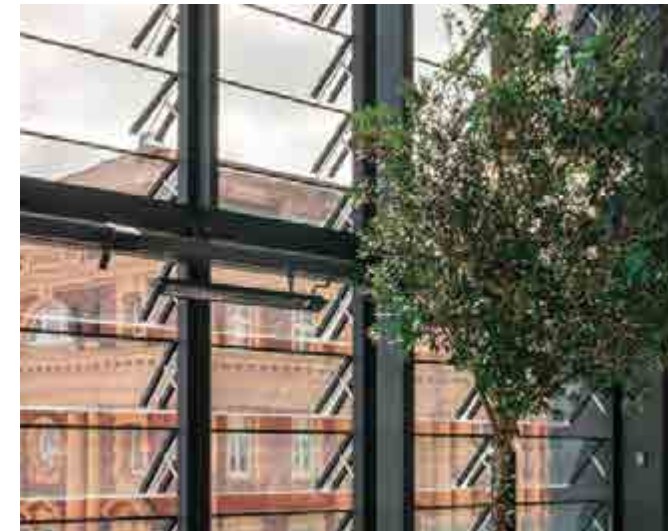
Operable louvres along the north and east facade of the café terrace will provide wind mitigation to the cafe balcony
