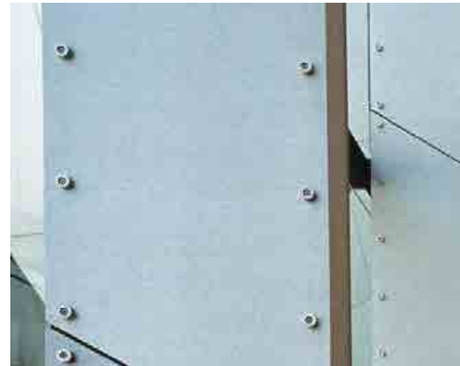
Aluminium panels with exposed fixings providing a textural material related to ground plane
